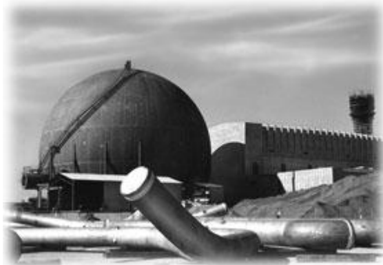
On the left is the gigantic sphere, which houses the nuclear reactor. On the right is the powerhouse to contain the generators and the water tower. In the foreground are the specially welded stainless steel pipers to convey steam from the reactor to the
