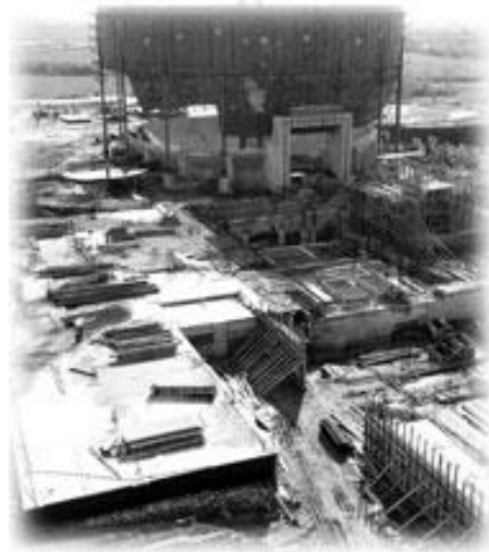
The photo shows the foundation of the giant sphere for the nuclear reactor in the background, 1960. Photo: SENN
