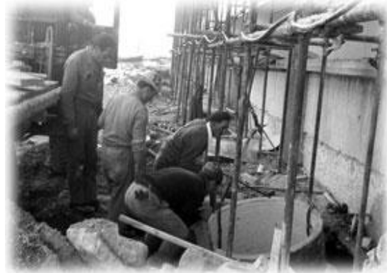
Italy's first nuclear power plant is under construction on the Garigliano River, March 1962.
