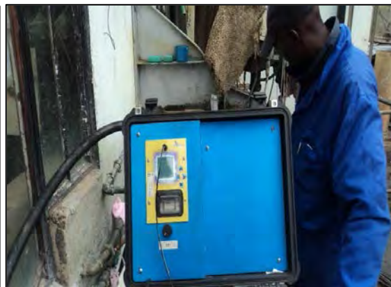
Testing of flow meter
