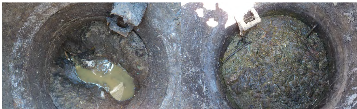
Sewer manholes blocked due to siltation in pipes
