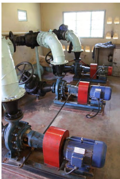
Mutare Road P/Stn: Existing Pumps to Elevated Tanks
