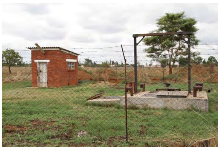
Narira Sewage Pumping Station
