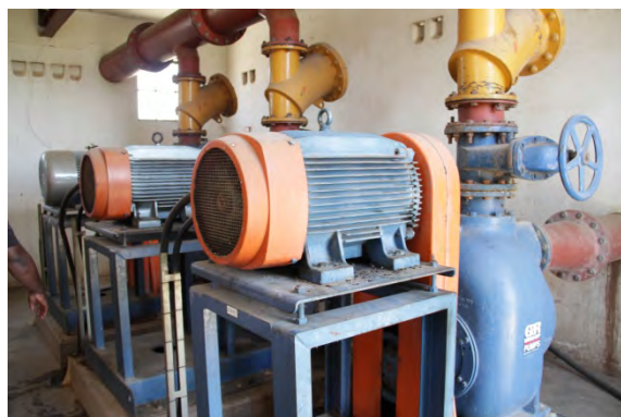
Ruwa Main SPS: Gorman Rupp Sewage Pumps
