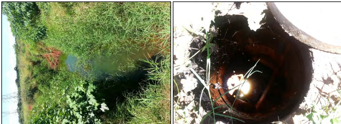
Collapsed section of the 600 mm Ø AC and state of Manholes on the main
