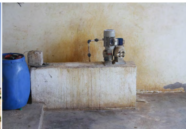
Ruwa WTW: Broken Down Chemical Dosing
