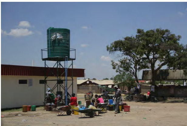
Water Point with Electric Borehole Pump
