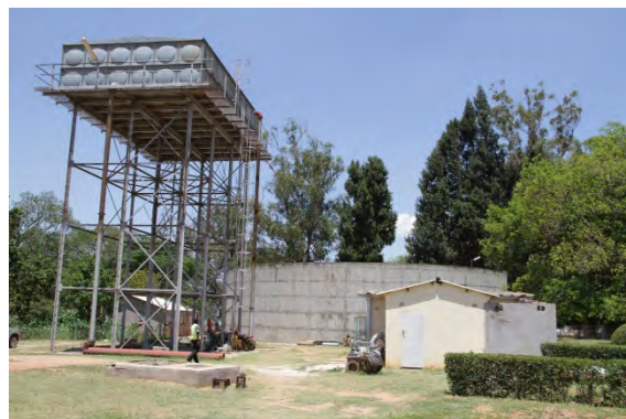
Mutare Road Elevated and Ground Tanks
