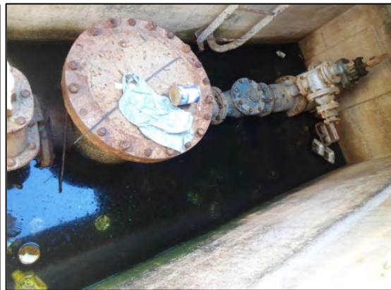
An off-take with faulty flow meter and PRV
