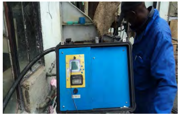
Flow meter testing
