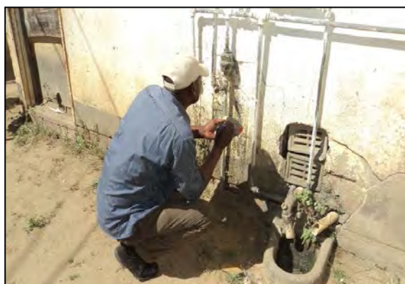
Testing of consumer water meter
