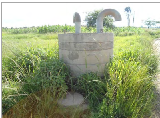
Air valve chamber along DN 1500 pipeline
