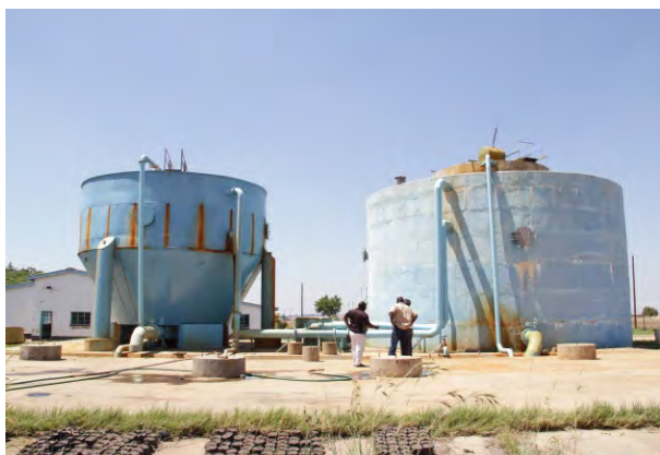
Ruwa WTW: FC Reactor Units 2.5MLD (left) and 5MLD (right)
