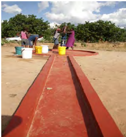
Water Point with Hand Borehole Pump
