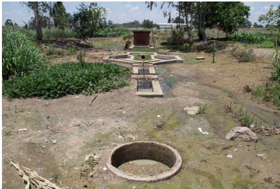
Relnyaro SPS: Intake works and sewage spills
