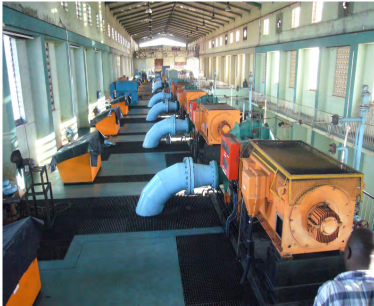
Treated Water Pump Station
