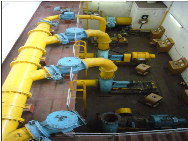
Low Lift Pump Station
