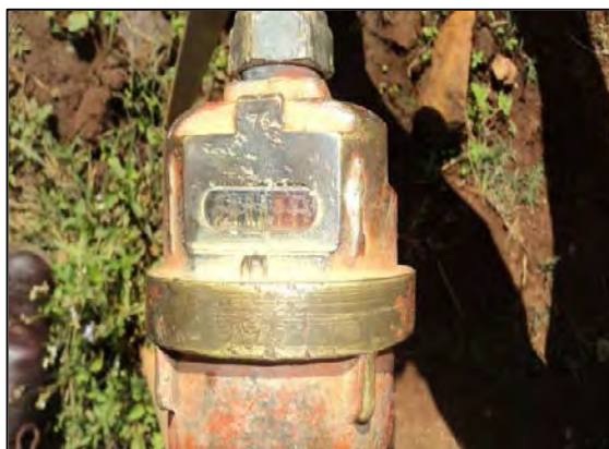
Vandalised water meter
