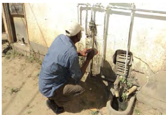
Water testing meter
