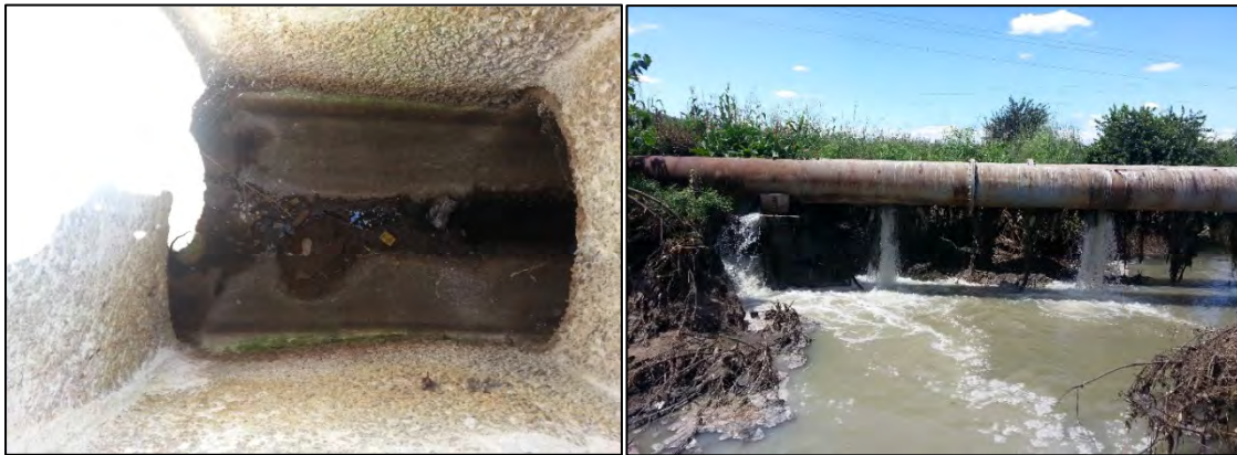
Condition of manhole and surcharging pipe on Pipe Bridge
