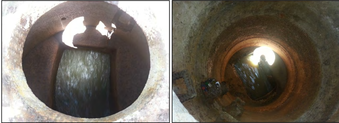
Condition of manholes on the 1400 mm Ø RC mains
