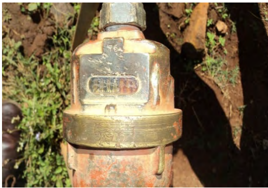
Vandalised water meter House connection
