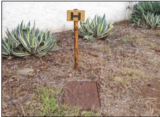
Fire hydrant chamber with marker post
