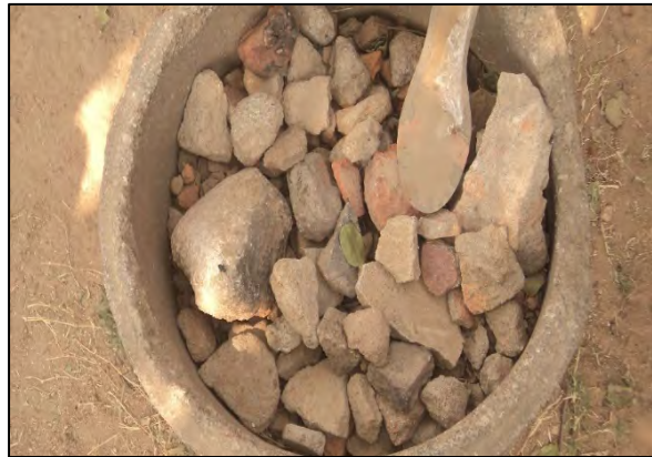
Valve chamber (vandalized)
