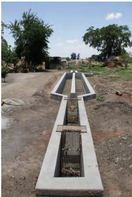
Chilemba SPS: Intake works
