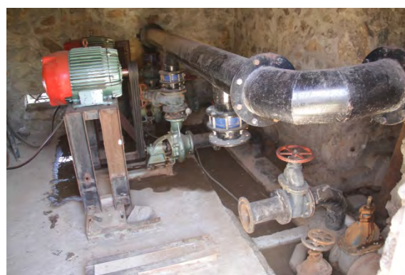
Green Sykes Raw Water Pump and pipework
