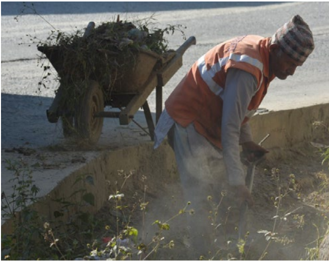
PLATE 1: The importance of routine maintenance cannot be over-stressed
