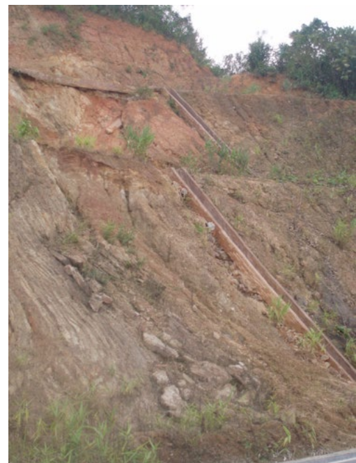
PLATE 4: This slope is beginning to deteriorate and could erode and fail without intervention.
