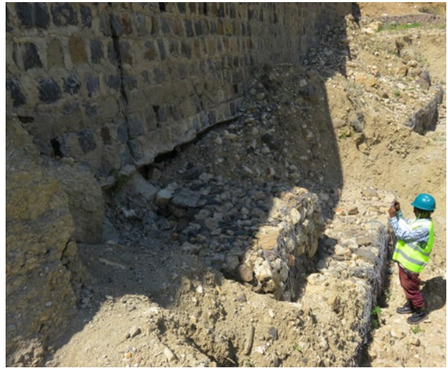
PLATE 2: Timely preventative interventions can avoid structural failure and loss of investment
