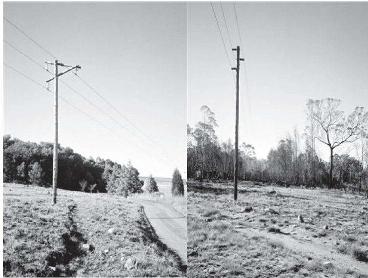
Picture A 2.1: 22 kV Rural Line. (Traditional Design on the left, New Design on the right)
