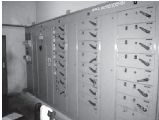
Picture A 9.1: Distribution Panel: Tanoso Waterworks
