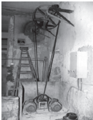
Picture A 1.8: Two Parallel Single-phase Motors Providing Additional Power for this Tunisian Industrial Client (Olive Oil Plant) (Cecelski, 2004)
