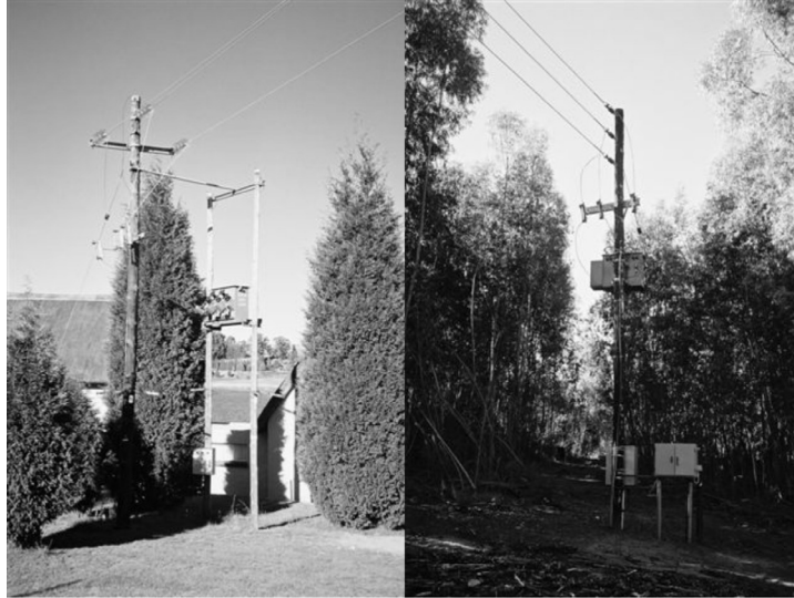
Picture 2.2: The transformer on the left is 50 kVA and the one on the right 100 kVA
