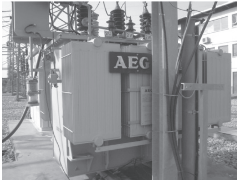
Picture A 9.4: Interposing Transformer at Techiman Substation
