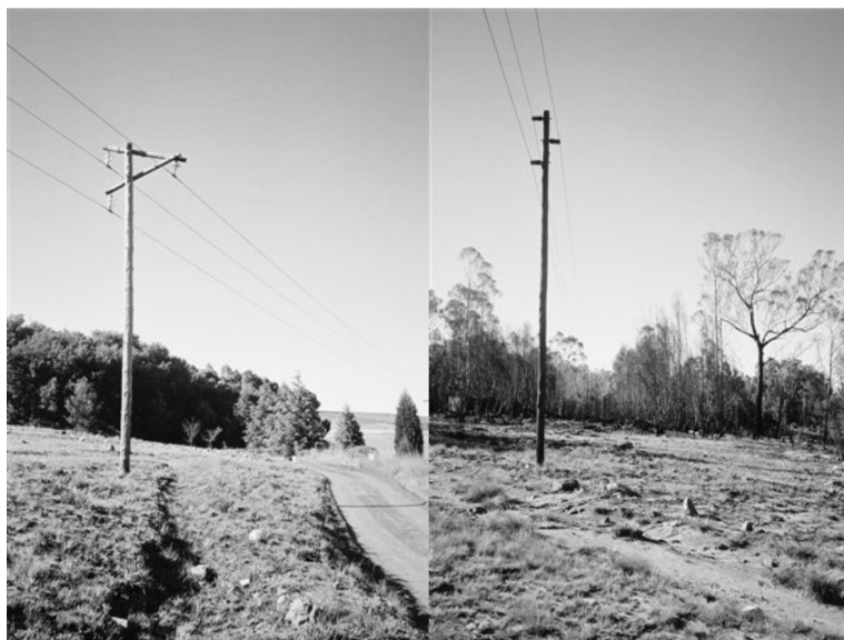
Picture 2.1: 22 kV Rural Line. (Traditional Design on the left, New Design on the right)
