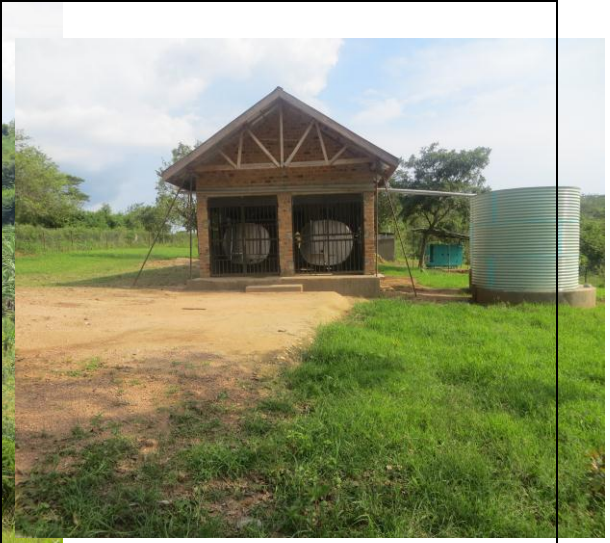
Figure 13: Milk Plant using a Diesel Generator
