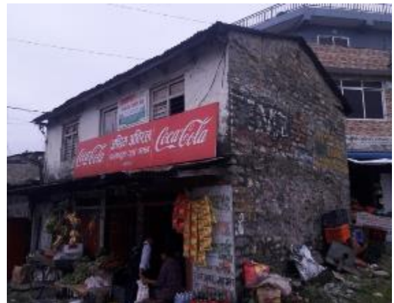
Road affected house at Sisuwachok
