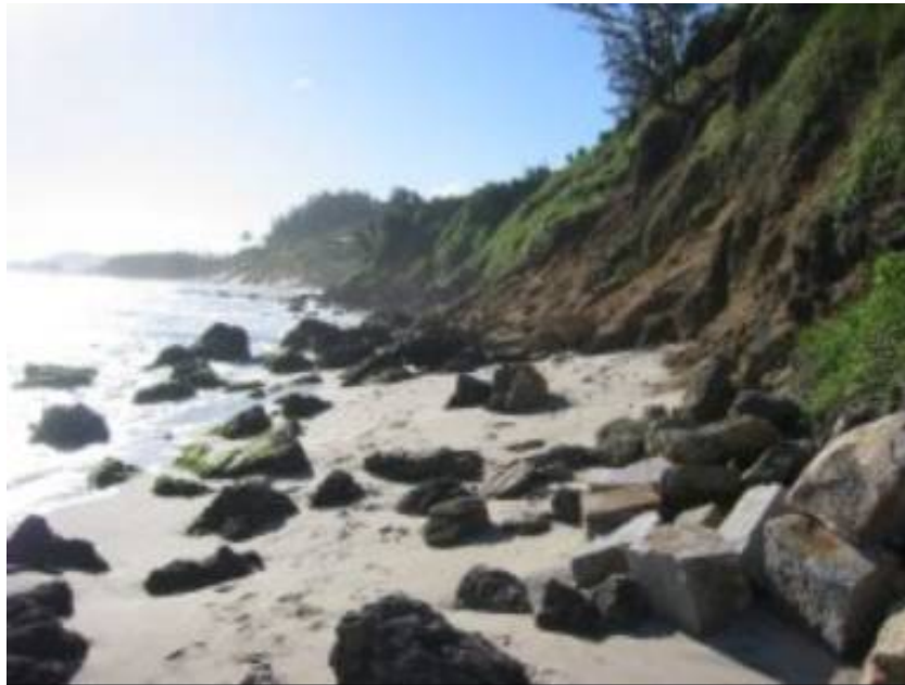
Figure 2.5 Shoreline Erosion at the North End of Fausse Baie des Galions
