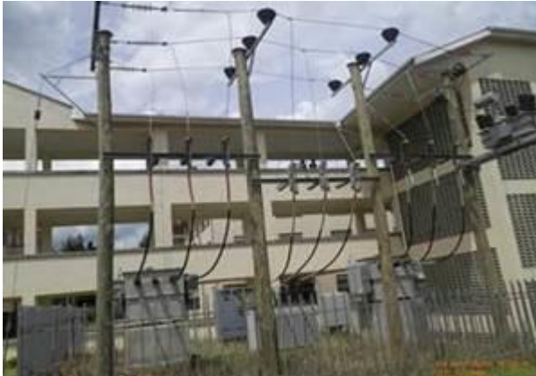
Photo 4.1: Grid power supply sub-station located in the hospital near the proposed project site
