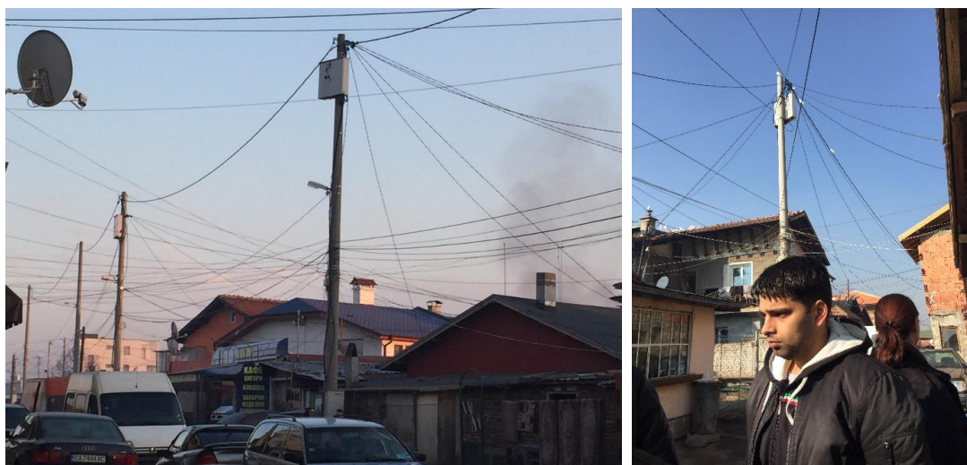
Plate 8.2 Individual electricity meters perched in boxes on top of electricity poles
