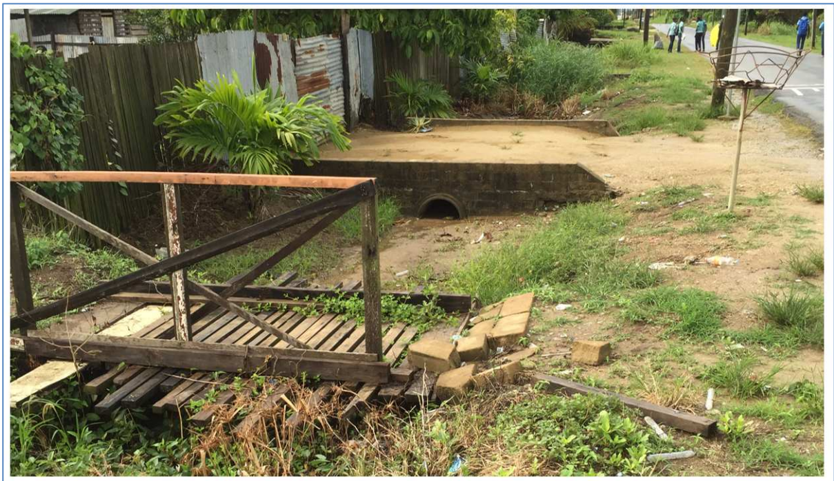
Figure 3-10. Sedimentation reducing conveyance on canal drainage system.
