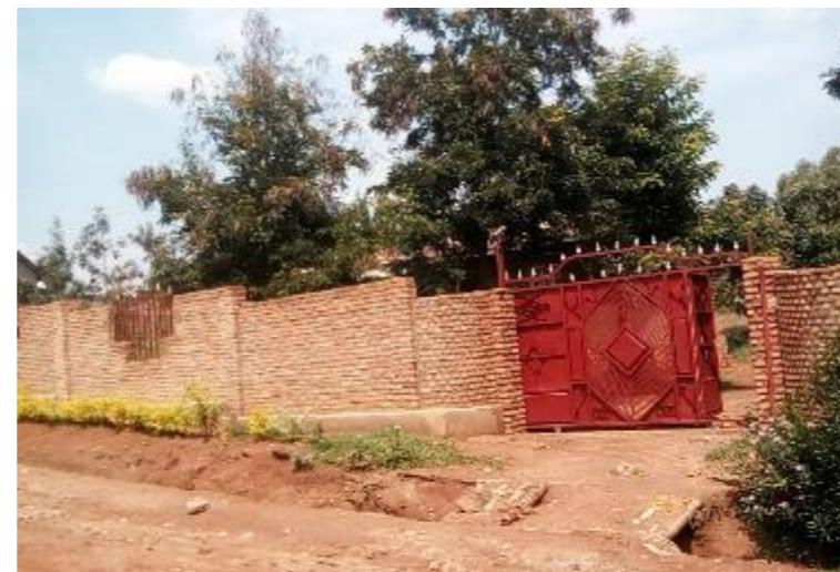
Affected boundary wall on RoW
