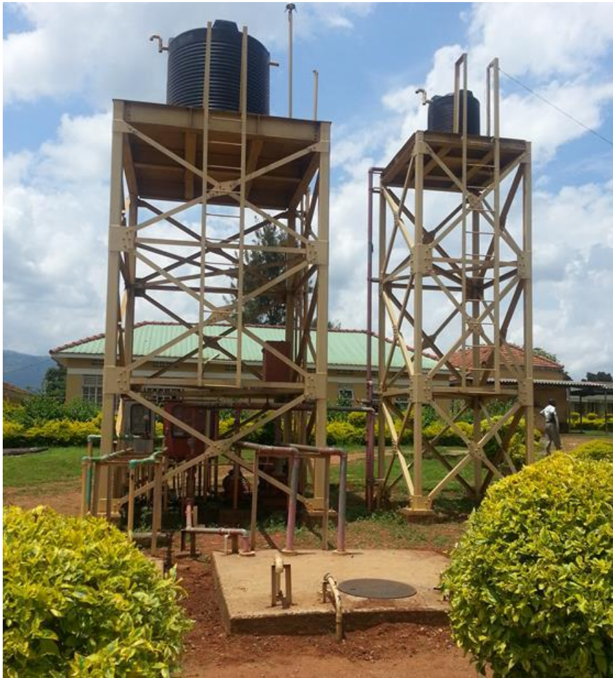
Photo 4.7: Groundwater supply system for emergency water supply to the ward of expectant mothers
