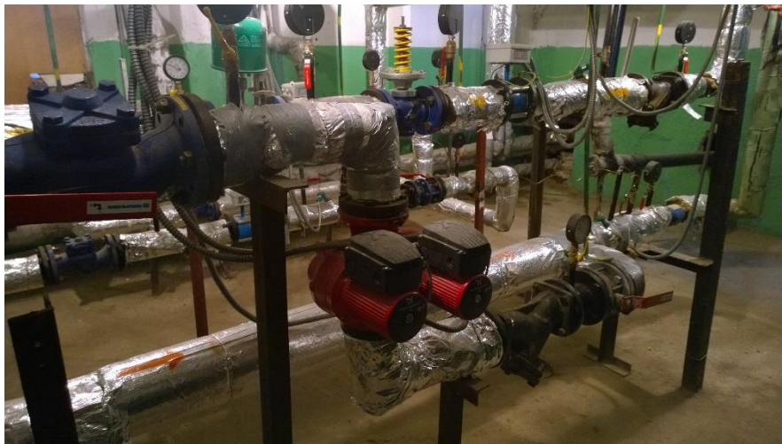
Figure 7: An existing mixing loop in Minsk with red twin-mixing pump in the center of Figure.
