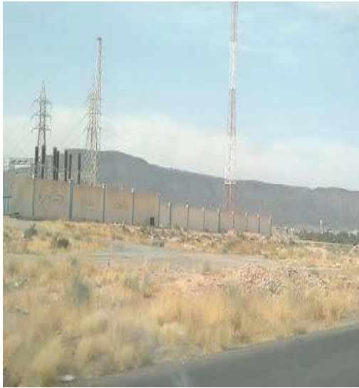
Figure 5-16: 220 kV Shakshuk substation
