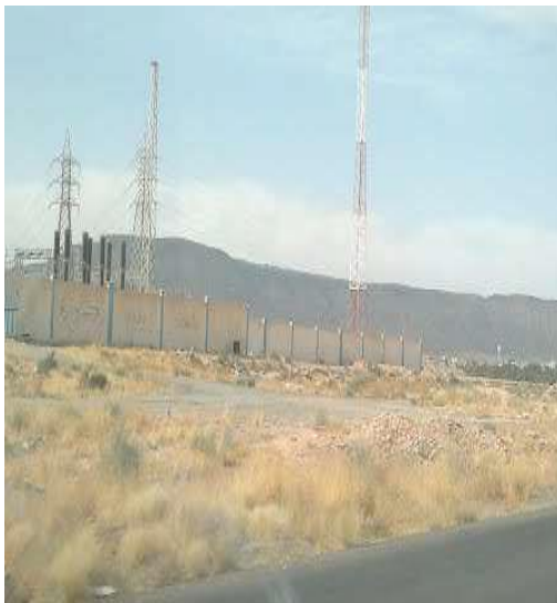
Figure 3-5: 220 kV Shakshuk substation
