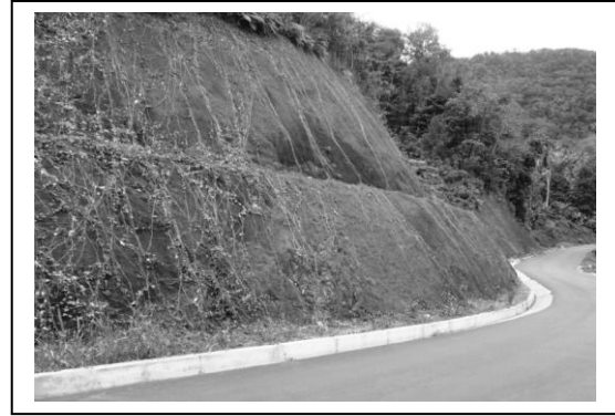
Example of lateral slope stabilization as applied on the rehabilitated road through the Central Forest Reserve
