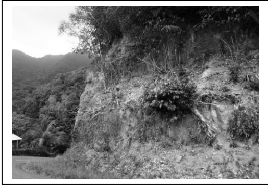
Other lateral escarpment in potentially unstable shape
