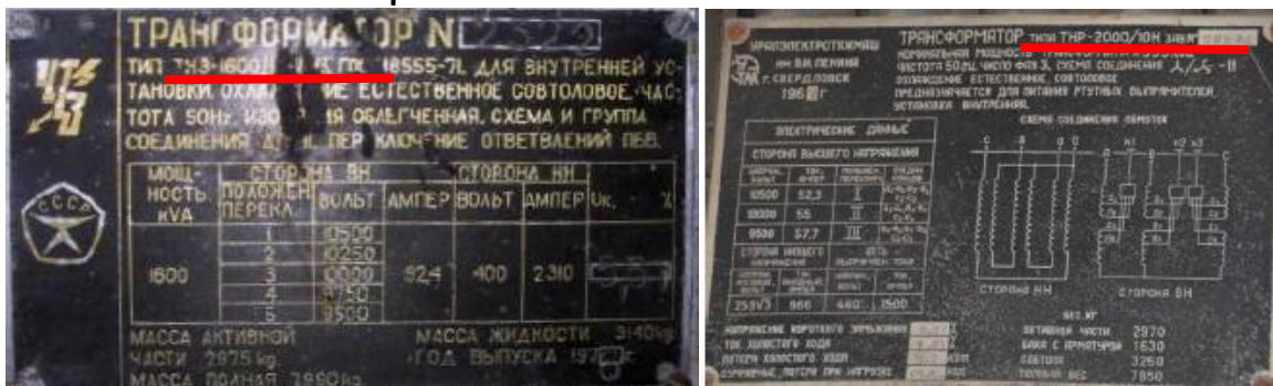
Picture 1: Manufacturer’s plate of Russian PCB transformers
