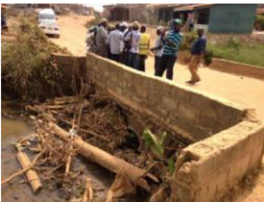
Pipe culvert blocked by debris
