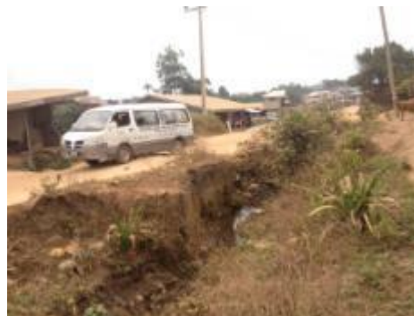
Collapsed culvert and road approaches without drainages
