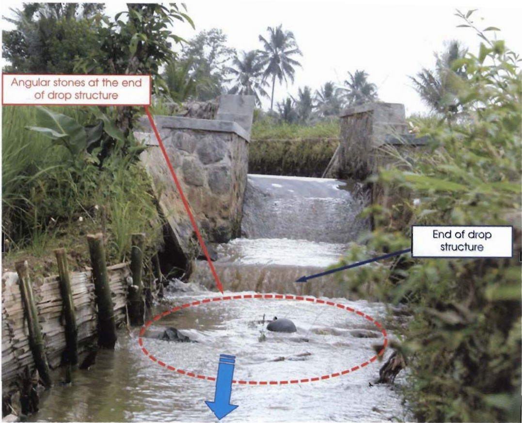
Protection of canal bed with large (angular) rocks Directly downstream from the concrete drop structure
