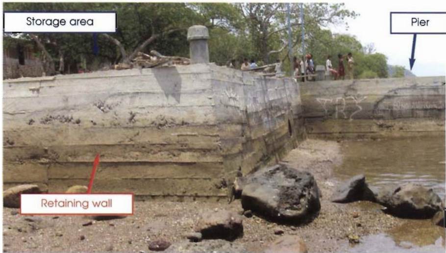
The concrete finish is unsatisfactory
