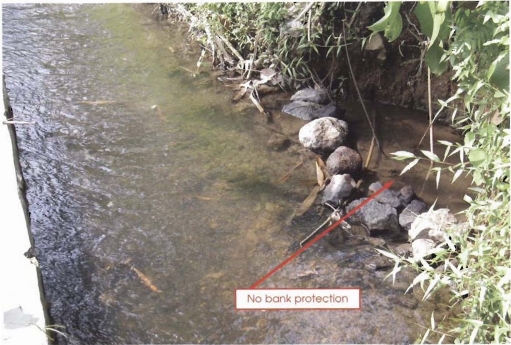
No protection against erosion, therefore the bank is washed out.
