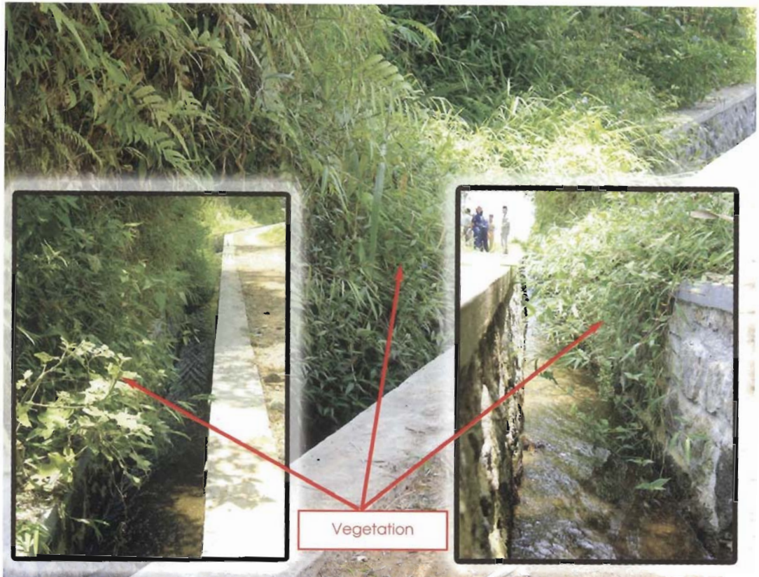
Vegetation growth can block the flow of water
