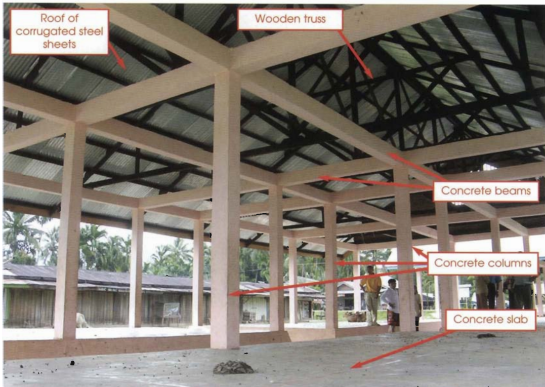
Market shed Type 3: Concrete columns and grid, wooden girders and corrugated steel sheets for the roof
