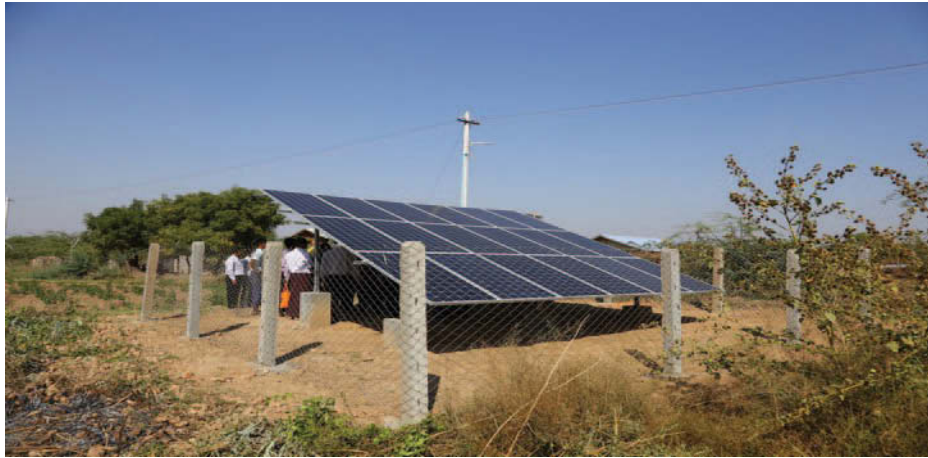
This 3.6 kW solar PV mini grid is one of three such mini grids in the village of Myin Chi Naing.
