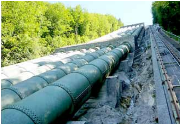
Figure 4-18: Steel penstock of the Walchenseekrafwerk (Germany)
