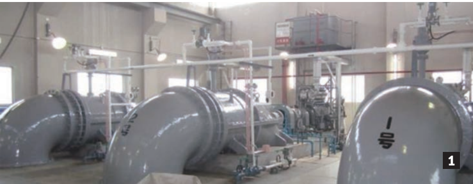
Figure A19.1: Storm Surge Measures in Kobe, —Iron Tide Gate, Flood Gate, and Pump Station Source: Takemoto 2019.
