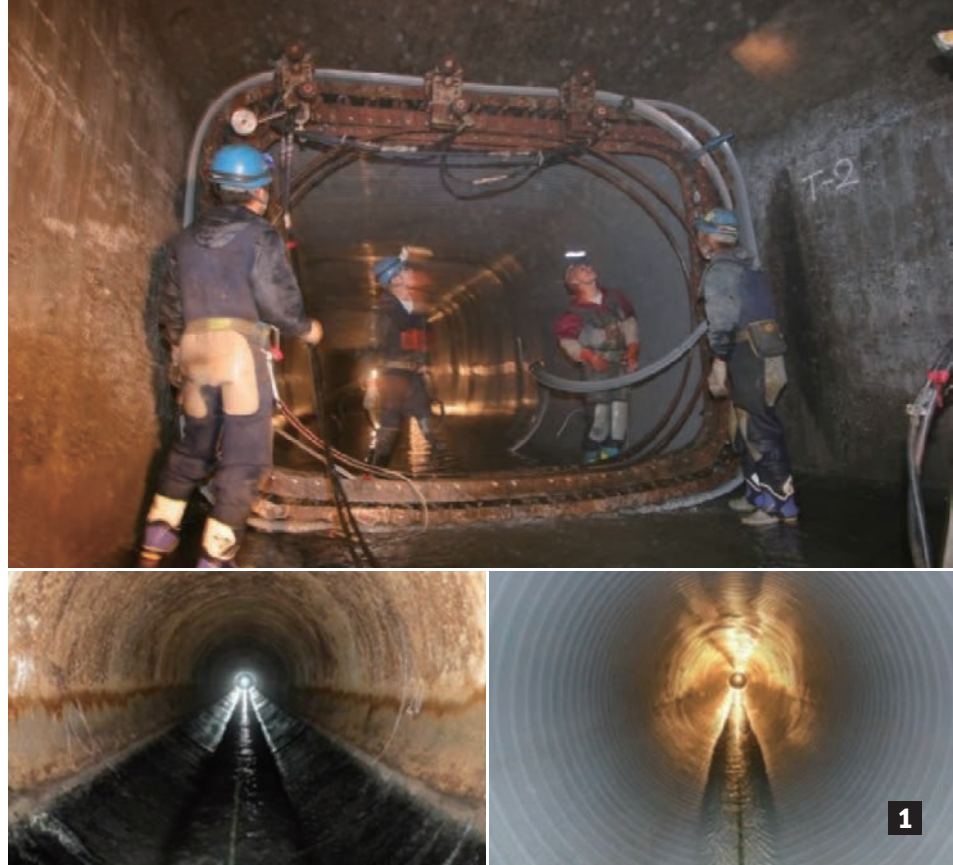
Figure A16.1: Renewal of Sewer Pipes (before and after) Source: Bureau of Finance, TMG n.d.
