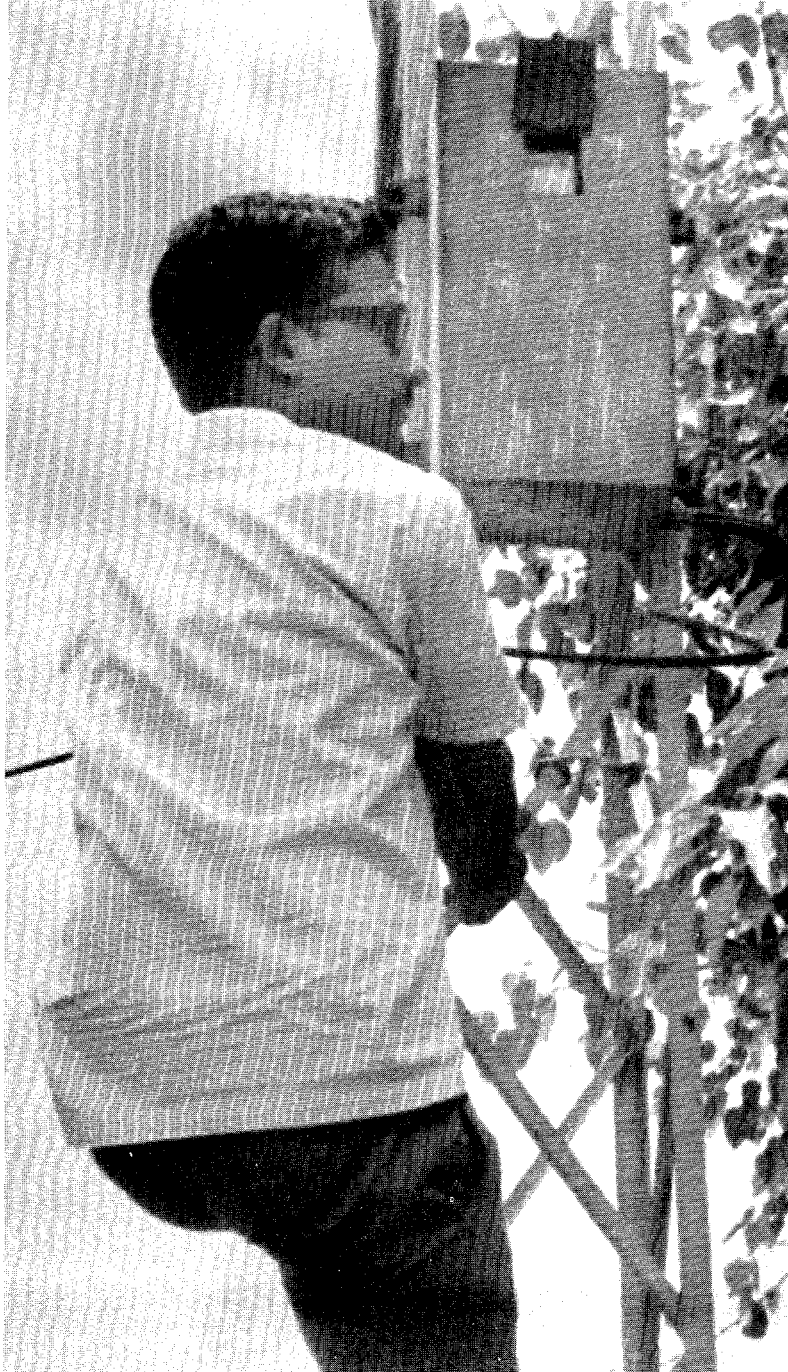
Figure 3.2 - This shows a steel box enclosing a meter serving a private tubewell. To read the meter (or to tamper with the box) it is necessary to climb the service pole.
