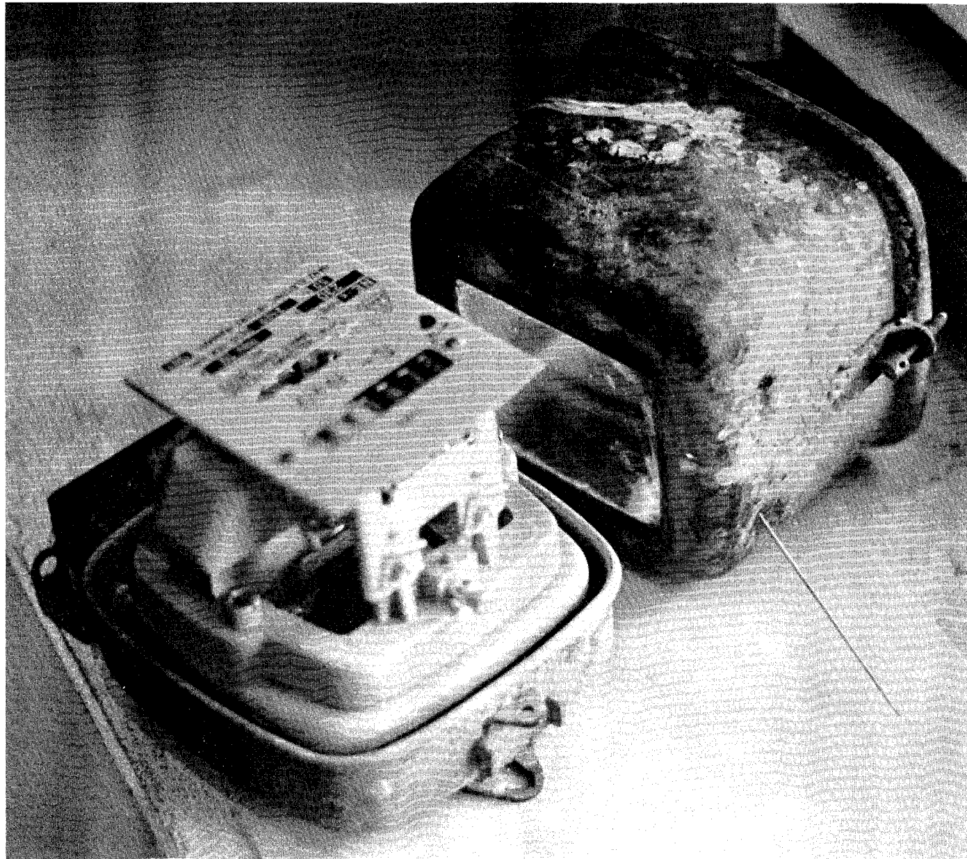
Figure 3.3 - The steel case of this single-phase meter has been pierced off-centre so that a needle may be inserted to brake the meter disc.
