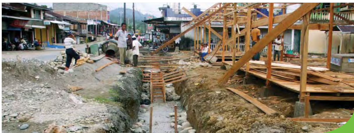
Construction has started on the section of IREP/IRFF supported national Road near Tapak Tuan. This is one of six sections of national roads (totaling 185 km) supported through IREP/IRFF which will link Meulaboh with Batas Sumut.
