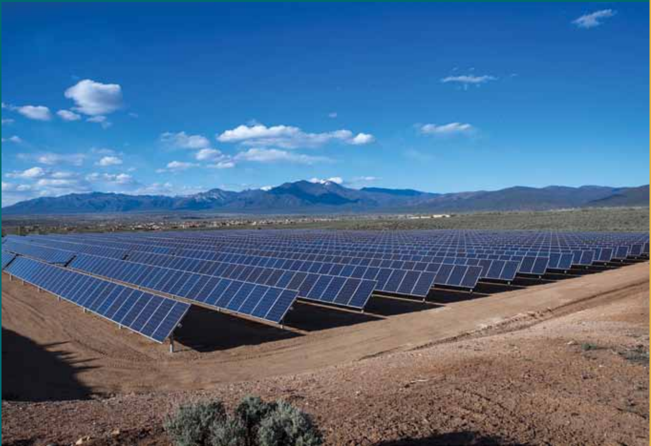
Figure 15: Large Scale PV Plant
