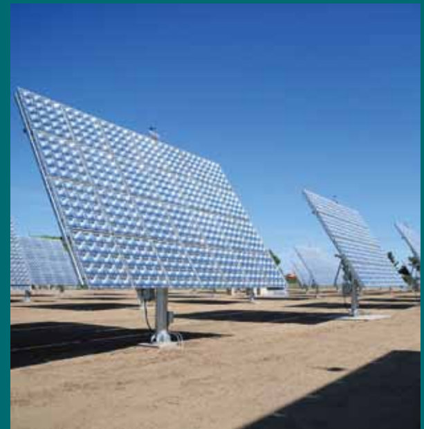
Figure 17: Example of SolFocus CPV Installation
