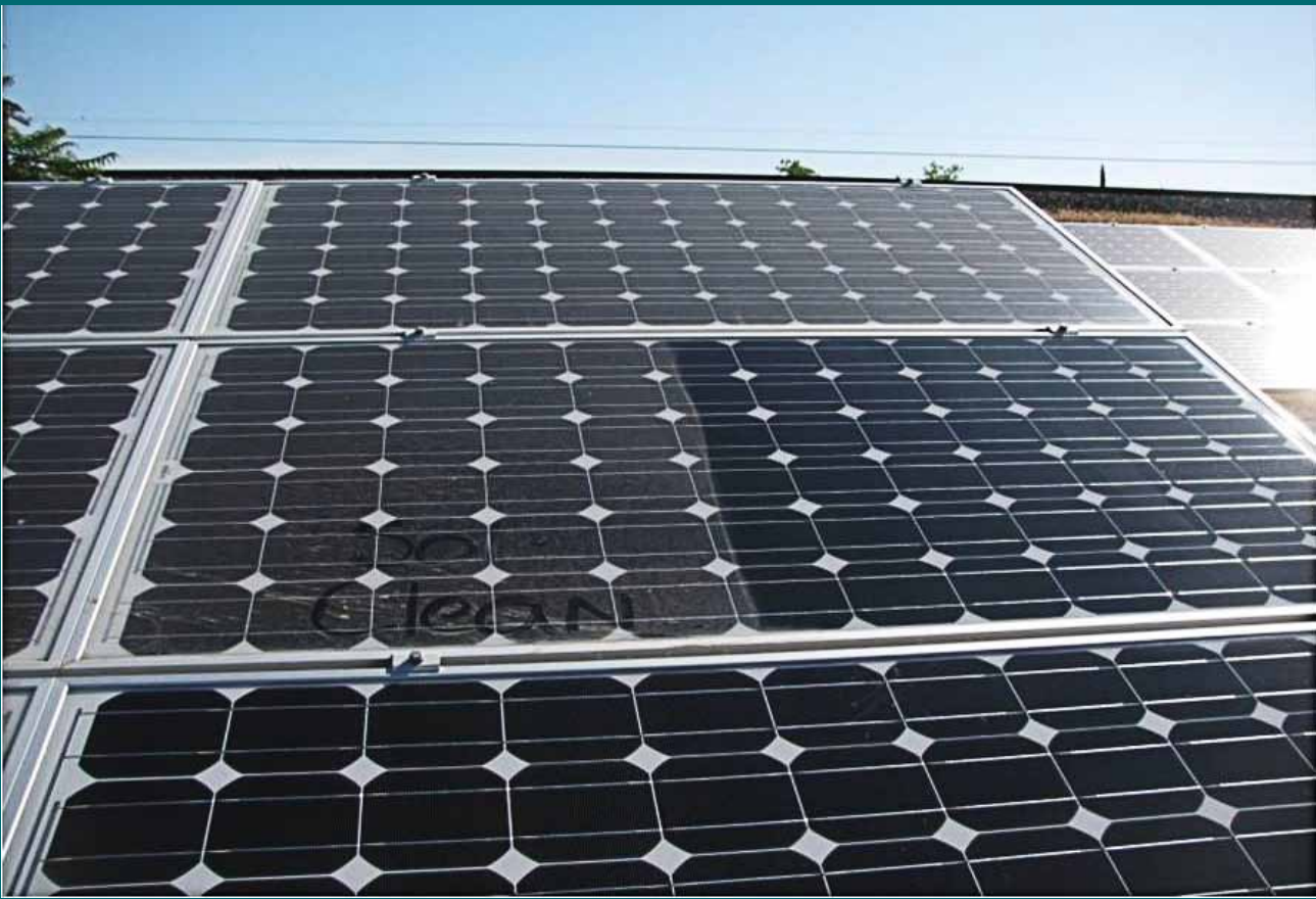
Figure 25: Solar Panel Covered with Dust
