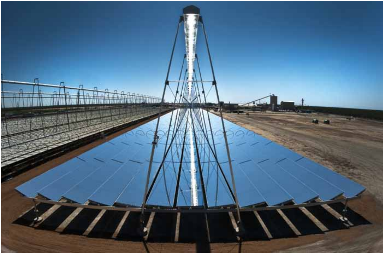
Figure 18: Kimberlina solar thermal energy plant, installed by AREVA Solar (USA)
