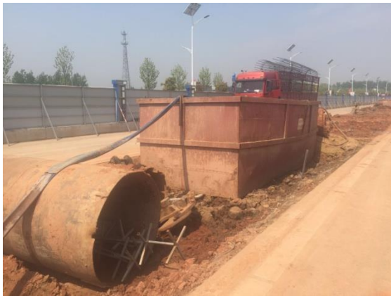
Slurry storage tank
