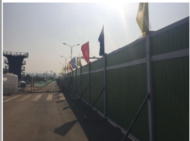
Spray system for dust control
