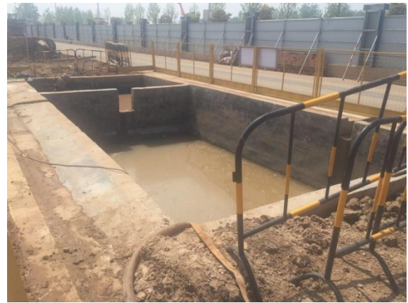
Three-stage sedimentation tank
