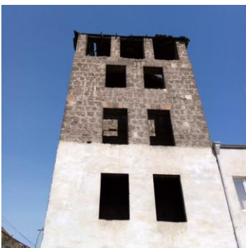
Training tower in FRS ID41 Vagharshapat
