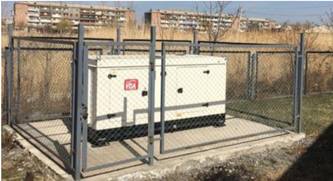
Figure 8.20: Emergency diesel generator in Artashat FRS
