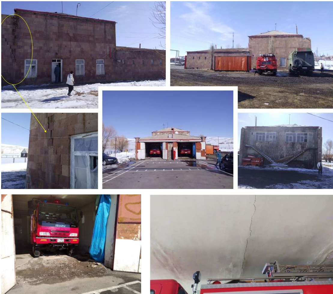
Figure 5.15: Two brand new mid-size ISUZU fire tenders housed in a degraded FRS building which barely fit in the garage – example from FRS ID11 in Ashotsk.
