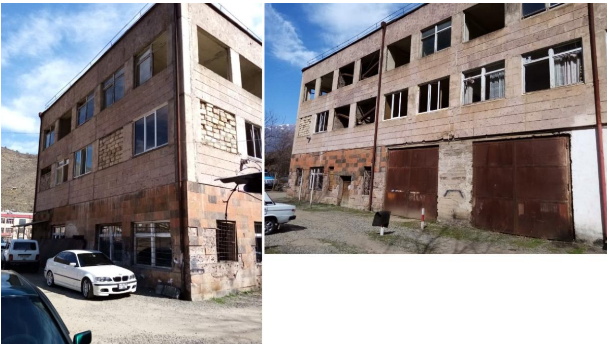
Figure 5.19: Lack of focus on regional centres - example of unused space and degraded building conditions in FRS ID52 in Kapan which share the building with the Regional ERC.
