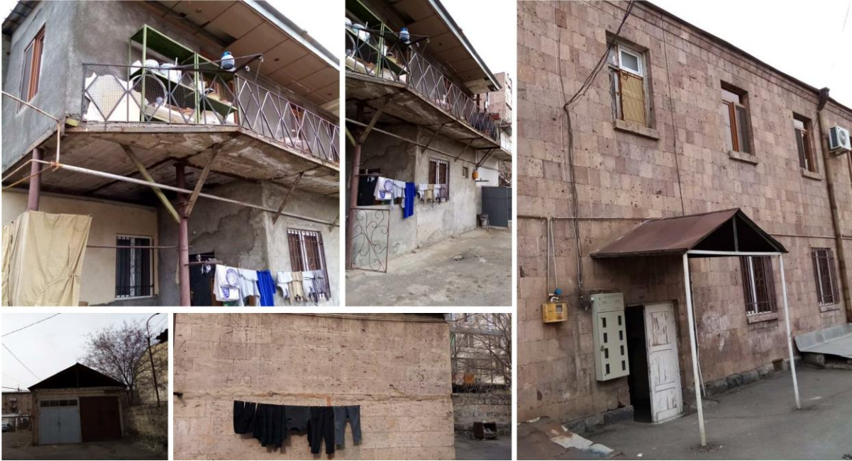
Figure 5.23: FRS which shares half of its 2 nd floor with private residents – FRS ID70 in Yerevan. Note, the nonengineered extension of the floor area made by the residents and the gas pipelines attached to the extensions making the building even more risky in a seismic event.
