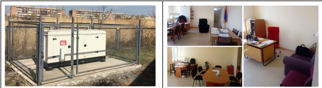
Figure 5.26: FRS in Artashat – improved interiors, installation of an automatic EDG (the only one within the portfolio of FRSs in Armenia).
