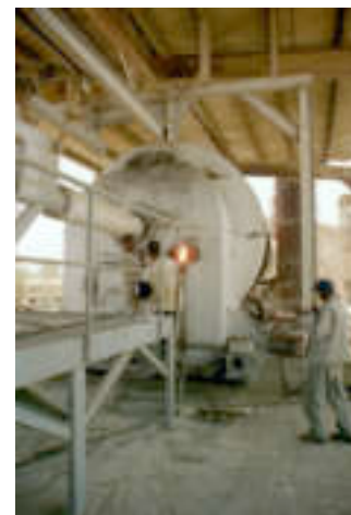
Photo 12: The rotary kiln at the Eritrean Cement Factory in Massawa
