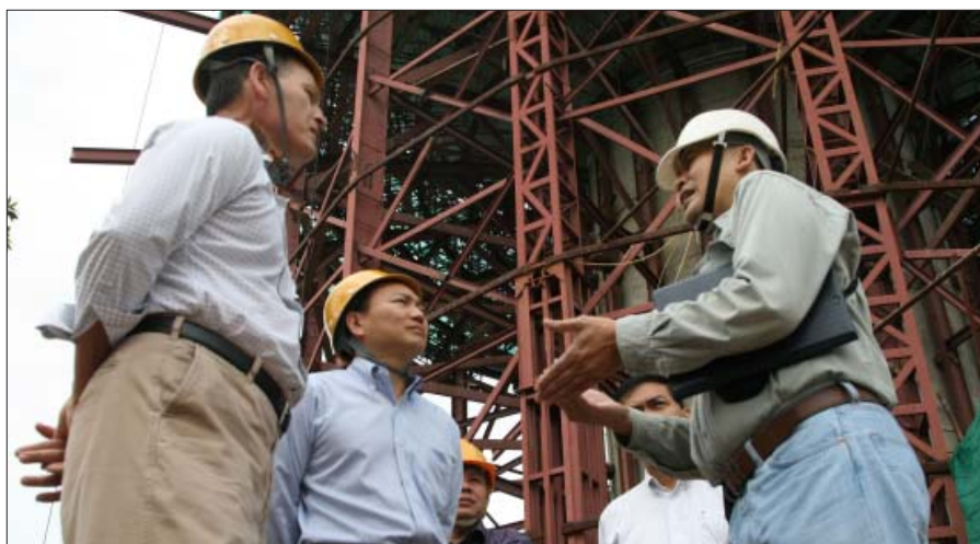
World Bank Executive Director Jim Hagan, left, discusses the Takmao water tower progress with Samrith Sovithea of the Phnom Penh Water Supply Authority, right.
