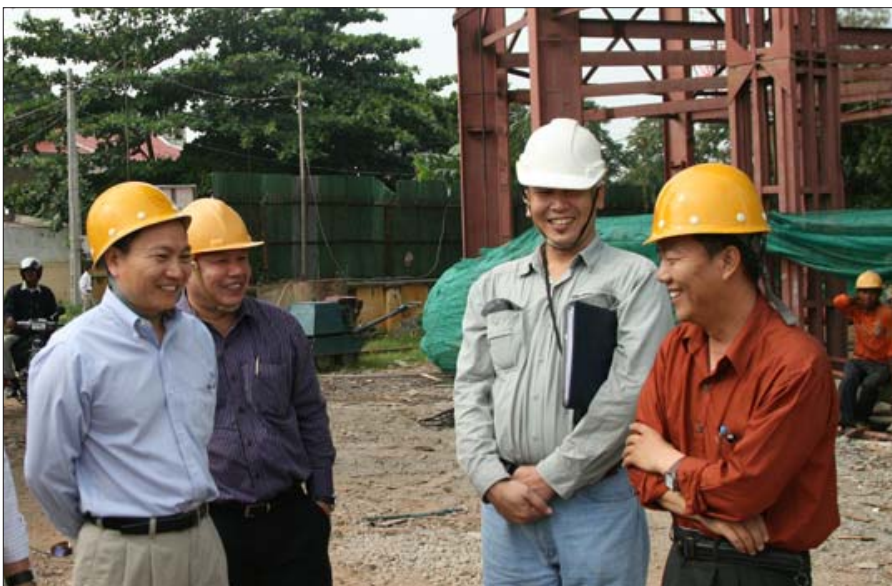
Mr. Fan talks with Phnom Penh Water Supply officer and private contractor to learn about progress of the water tower construction in Takmao town.
