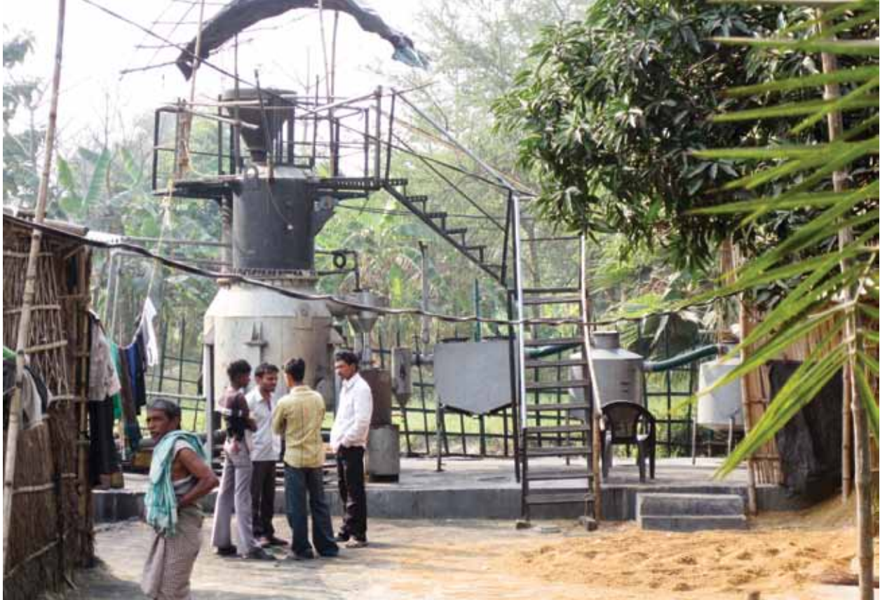
Husk Power Systems Biomass minigrid in Bihar, India
