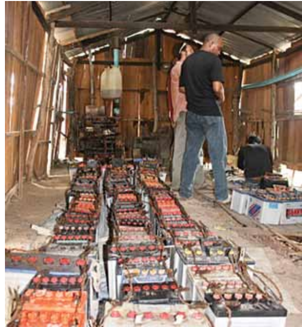
Battery Bank in Cambodia Image courtesy of Kamworks
