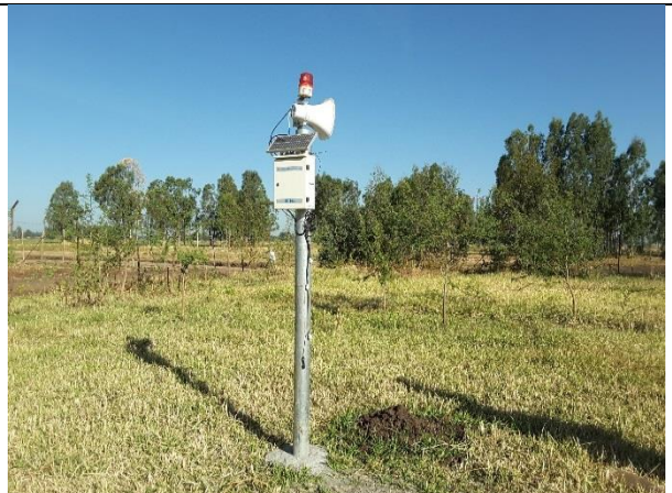
Flood warning sirens
