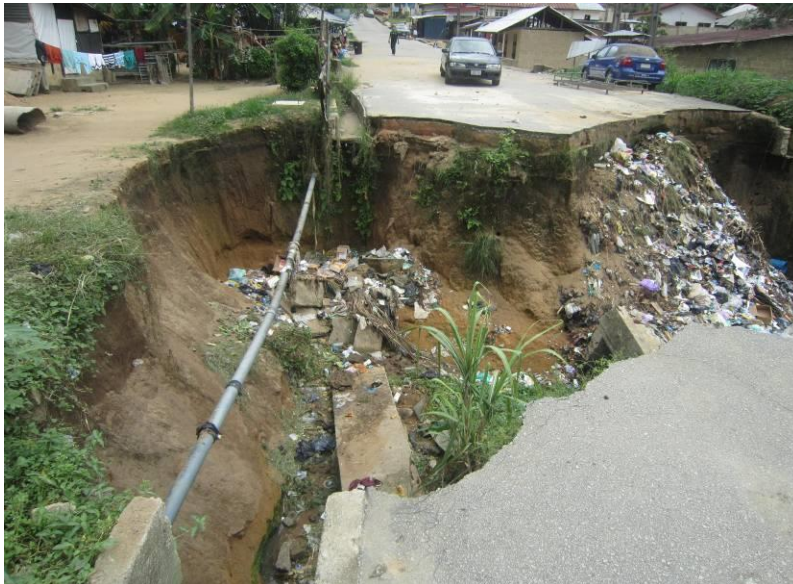
Plate 1.5: Command area of gully site at Ekorinim II (Gully Finger No. 5). The road has been severed and water pipelines exposed).
