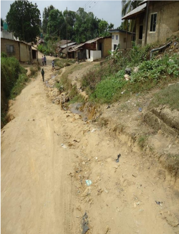
Plate 4.2: An eroded access road in Ikot Anwatim.
