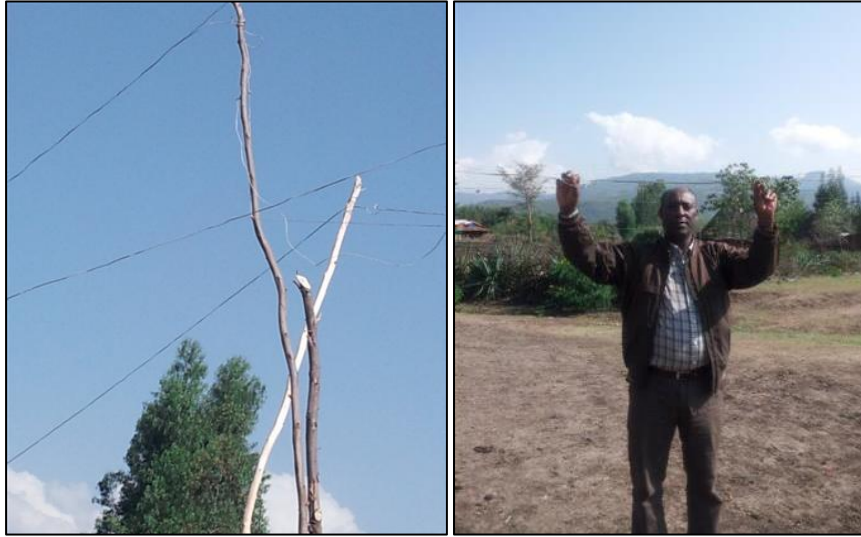
Figure 3.4 Poor Installation Procedures for Indirect Electricity Connections in Ethiopia
