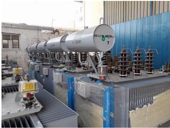
Item No 8 in the warehouse: 1000KVA Outdoor Distribution Transformers
