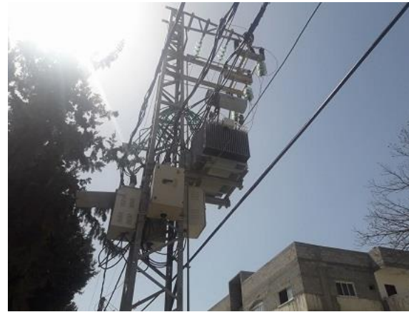
1000KVA Distribution Transformer installed in in North Gaza
