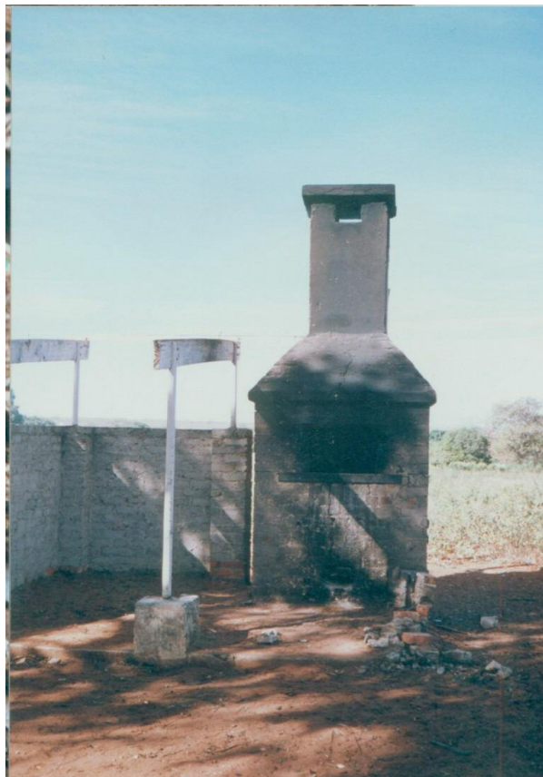
Picture 12: Unprotected incinerator at Livingstone general hospital
