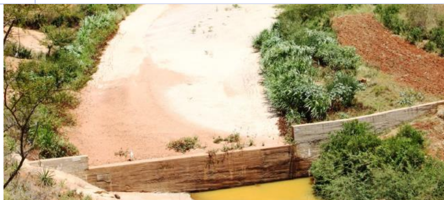
Figure 27: Aerial view of a Sand Dam in Kenya (photo courtesy of: Excellent Development)
