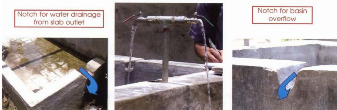
Hydrant and details
