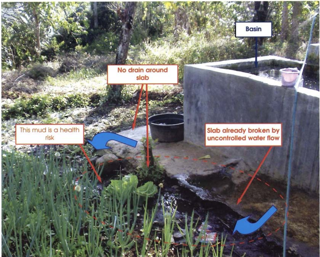
Spilled water is not drained to a ditch Slab washed out because of uncontrolled water discharge
