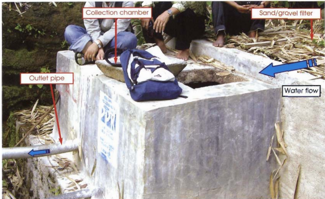
Collection chamber for a spring with sand/gravel filter
