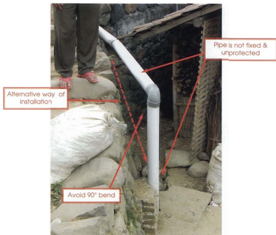
The pipe can easily get damaged
