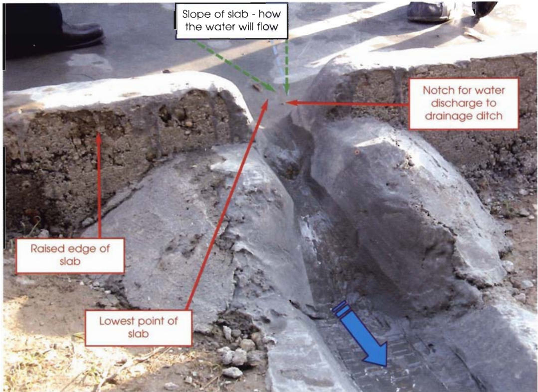
Notch for water discharge to a drainage ditch from a sloped slab around tank
