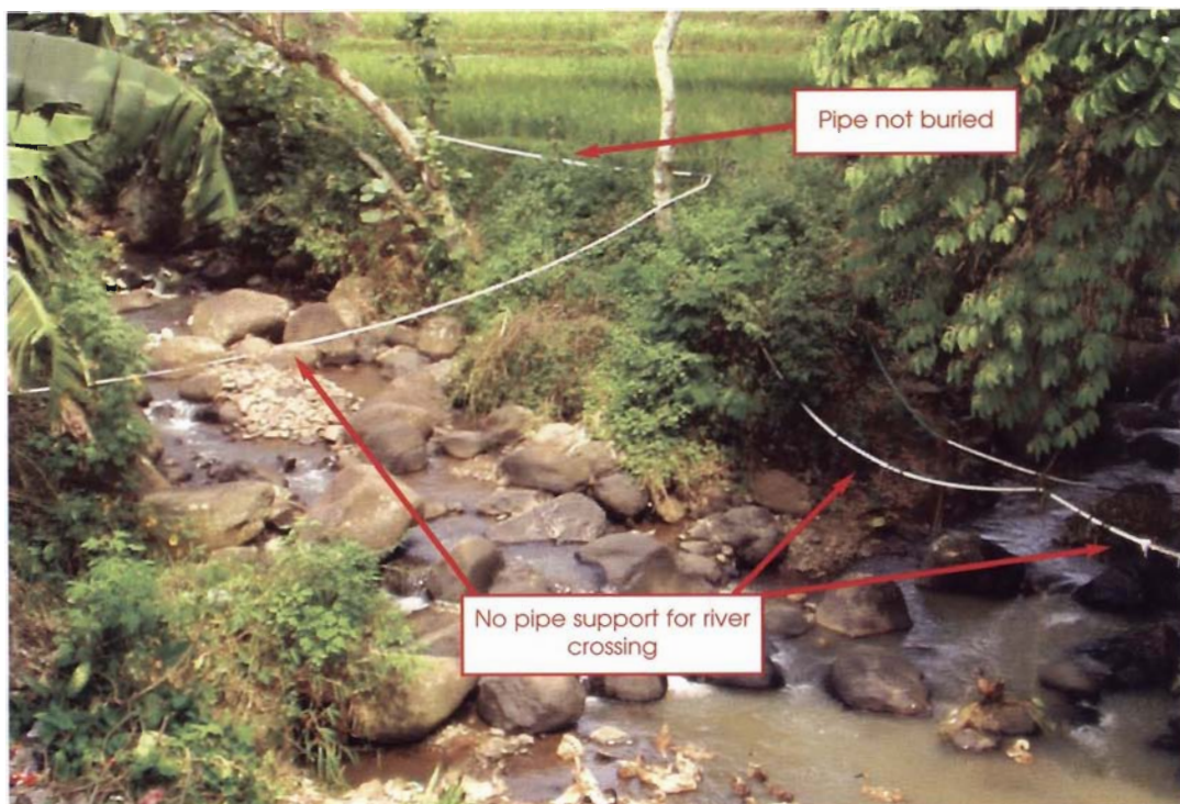
The pipes sag if a river is crossed without any support And they are exposed to flood water damage
