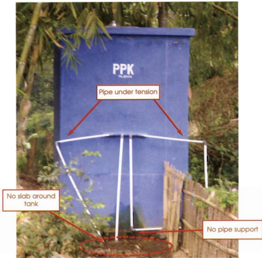
Pipe is under tension stress No pipe support at the bend
