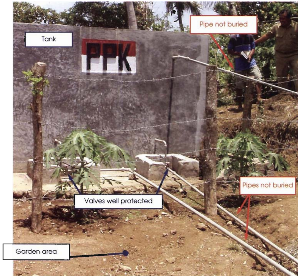
Pipes can easily get damaged
