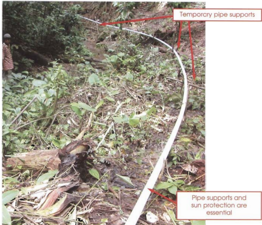
No permanent pipe supports - Pipe is not even buried No protection against sun
