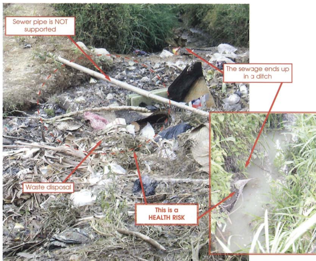
This is not an acceptable way to discharge a sewer!
