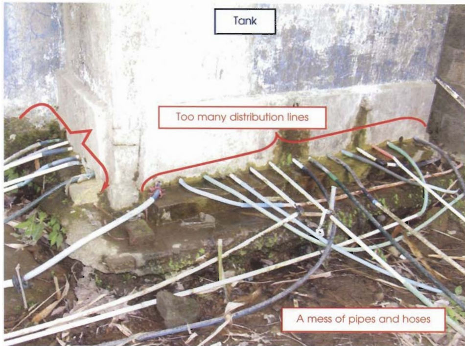
.Too many pipes & hoses need too many holes in the tank
