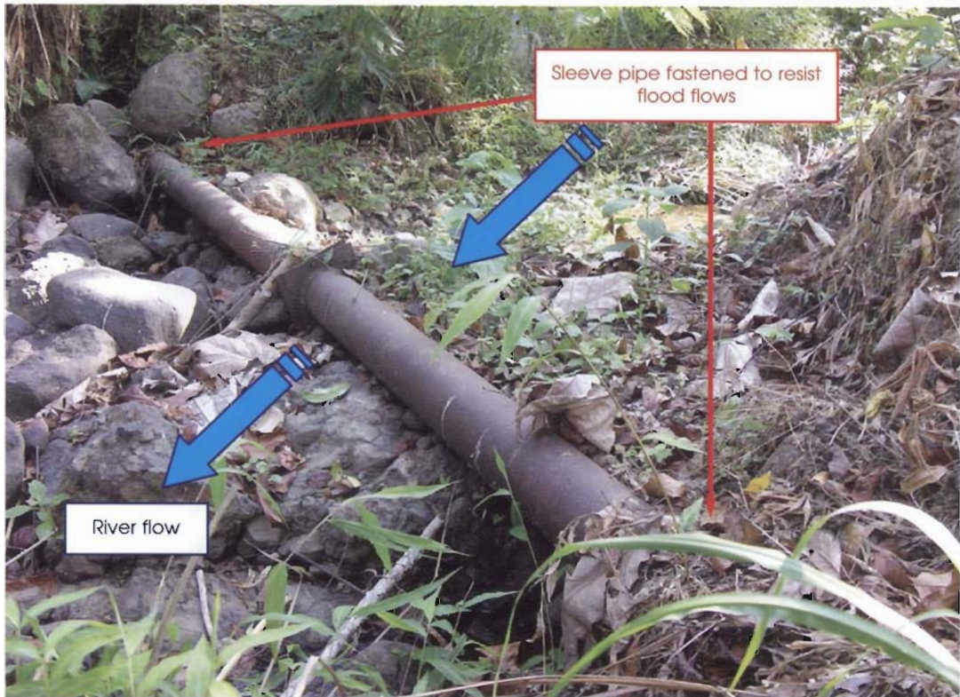
Pipe sleeve used for a river crossing
