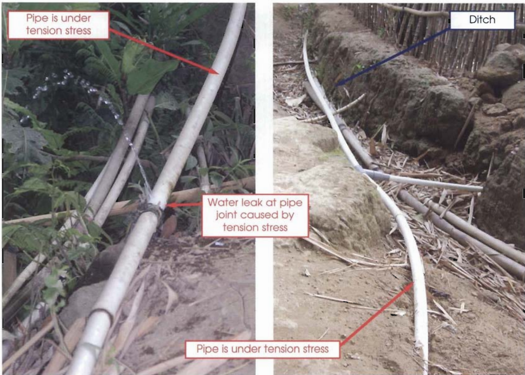
Pipes are improperly installed and not protected against damage
