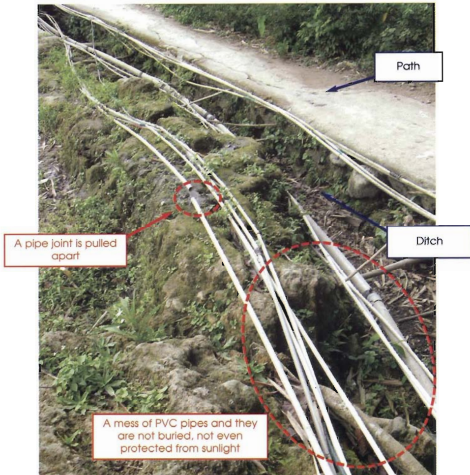
Distribution pipes are not laid in common trench Pipes are not protected against damage or UV-rays from sun
