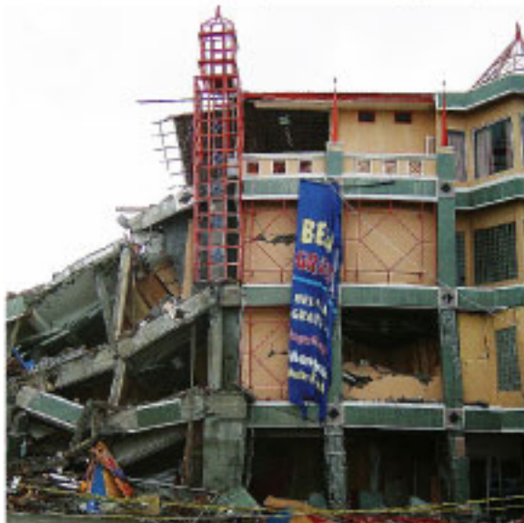
Earth Quake Damage, Leveling Shops
