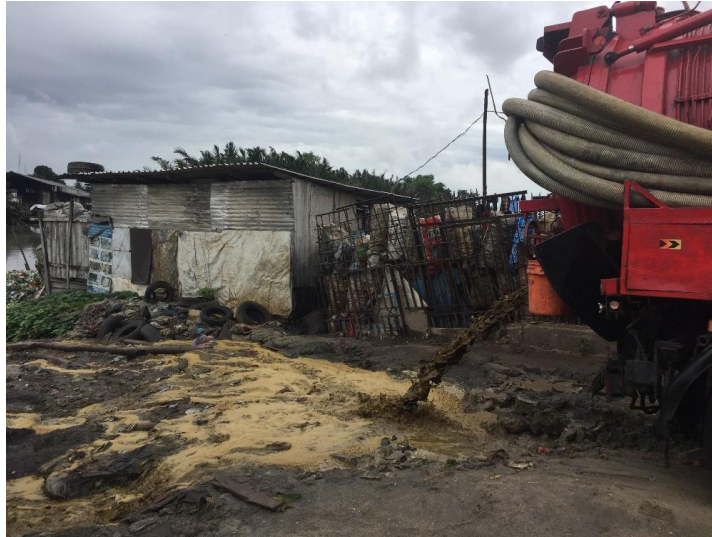
Figure 9: Excavator truck emptying fecal sludge directly into the river at the Amadi Ama dumpsite
