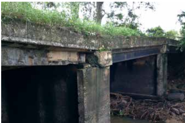
Weak bridge to be reconstructed, Batticaloa, Sri Lanka Photo by: Suranga Kahandawa
