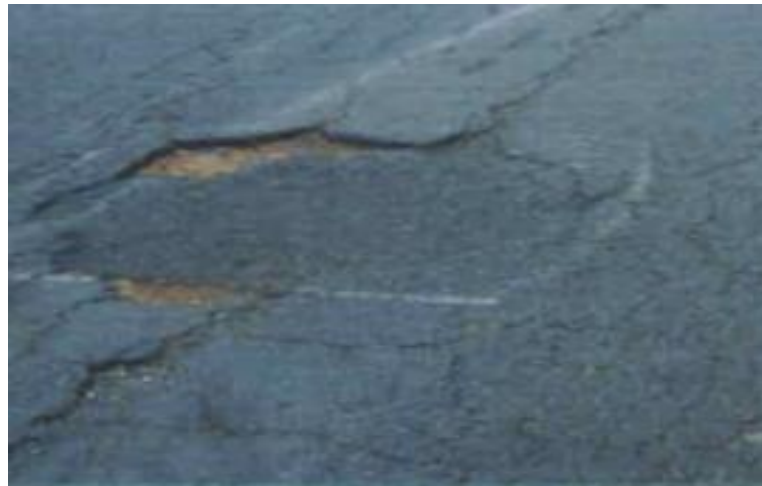
PHOTO 18 : REPARATION DEGRADEE (RN2)
