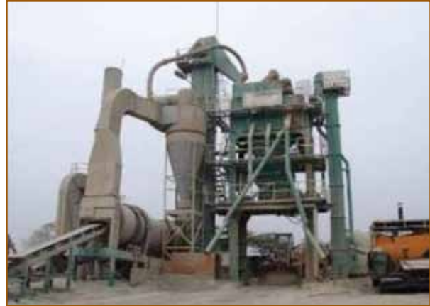
Modern Asphalt Plant near Hanoi, Vietnam
