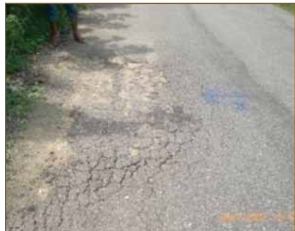
Pavement Surface Fatigue on Provincial Road in Indonesia
