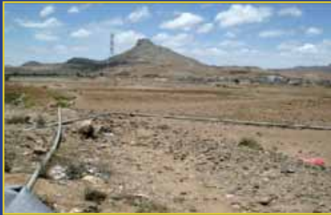
Water pipes in Qa' Al Qaidi
