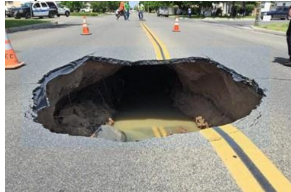
Sinkhole triggered by a heavy rain (California, USA)
