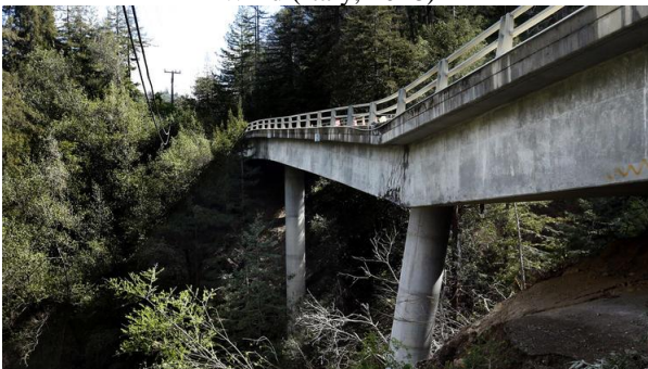
Landslide (California, USA, 2017)
