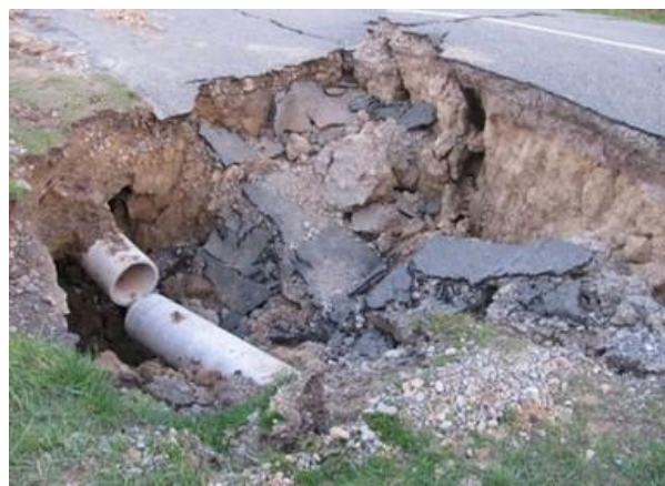
Liquefaction (pipe break)
