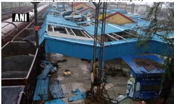
Wind (roof and wall damage)
