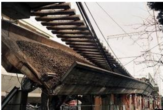
Earthquake (bridge pier collapse)
