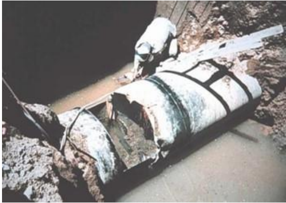
Earthquake (joint failure; Mexico City Earthquake, 1985)
