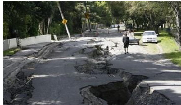
Liquefaction (Chirstchurch, New Zealand, 2011)
