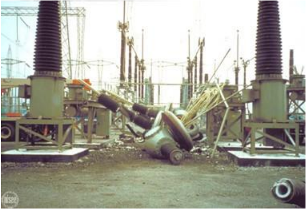
Earthquake (Northridge Earthquake)
