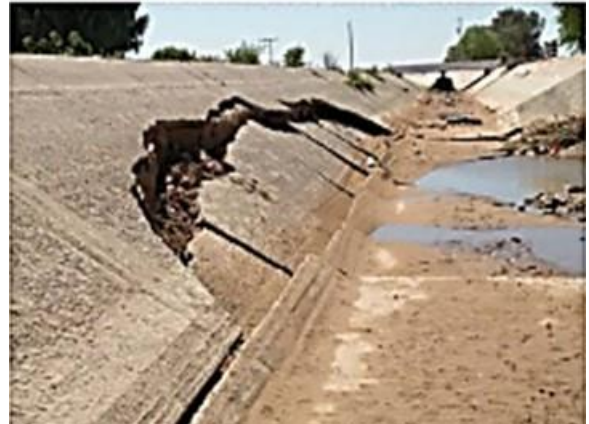
Liquefaction (Mexicali, Mexico, 2010)
