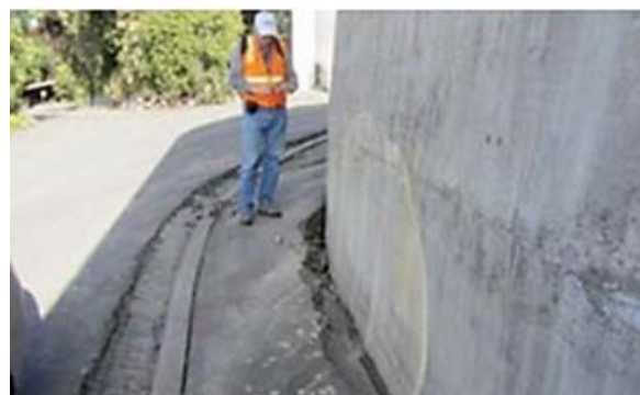
Liquefaction (2011 Christchurch Earthquake)
