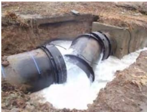
Earthquake (pipe joint pullout)
