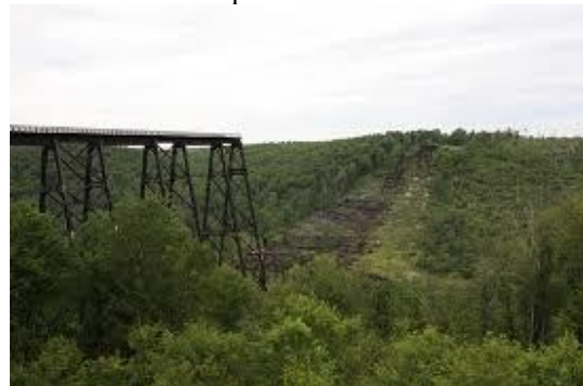
Long-period and multidirectional wind damage
