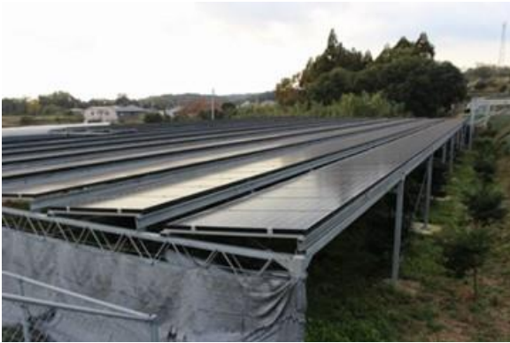
Earthquake (Kumamoto Earthquake, foundation slide)
