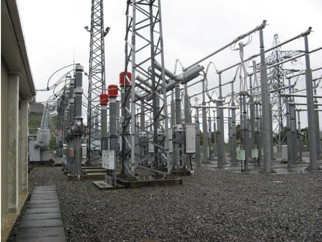
Figure 31. High-voltage electrical substation
