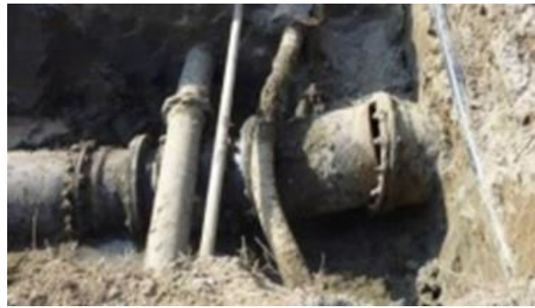
Liquefaction (break of a buried pipe)
