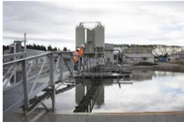
Liquefaction, wastewater treatment plant (New Zealand)
