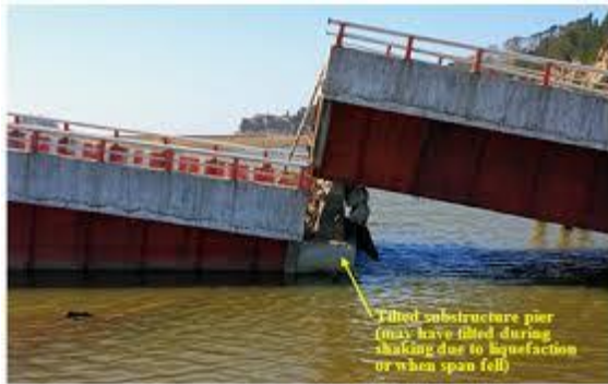
Liquefaction ground-movement damage
