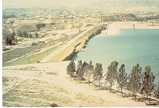
Liquefaction (1971 San Fernando Earthquake)
