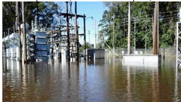
Flood (aftermath of Hurricane Matthew)
