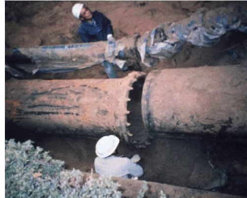
Liquefaction (pipe joint pullout; Kobe, Japan, 1995)
