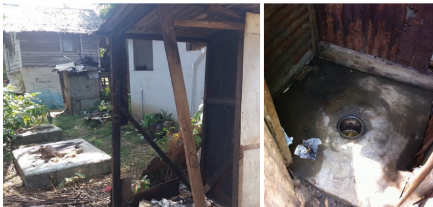
FIGURE 3.10: CLUSTER OF FUNCTIONING AND CLOSED PIT TOILETS IN BURNS CREEK NEAR HONIARA
