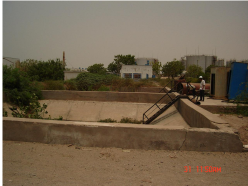
Figure-4.1.4 Sludge Drying Bed
