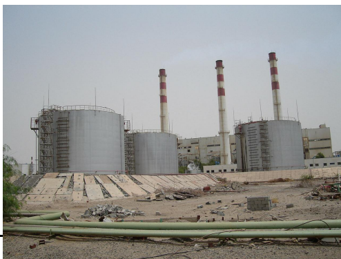
Figure-3.2.4 Fuel Oil Storage Tanks
