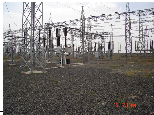
Figure-3.3.5 Existing 132 KV Dhamar Substation
