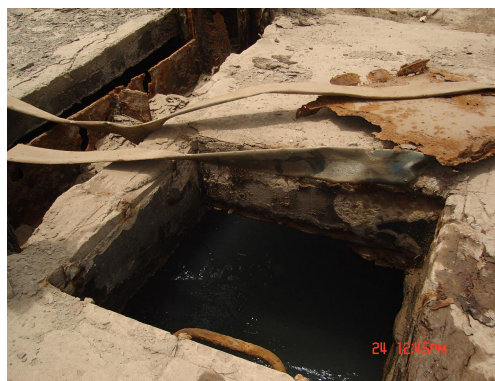
Figure-4.1.2 Oil Water Separator
