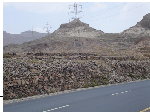
Figure-3.3.8 Existing 132 KV Dhamar-Sana'a Transmission
