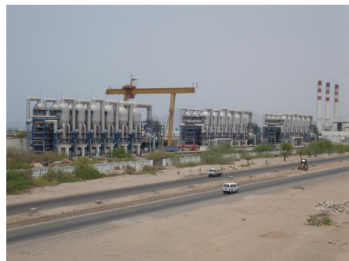
Figure-3.2.3 Desalination Plant
