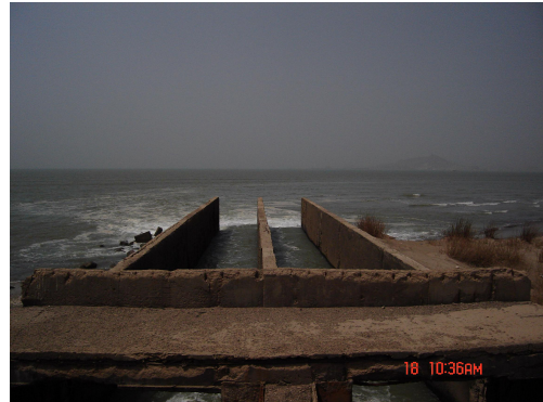
Figure-3.2.10 Cooling Water Discharge into Sea through
