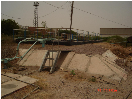
Figure-3.2.11 Sewage Treatment Plant
