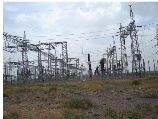
Figure-4.3.3 Existing 132 KV Dhamar Substation
