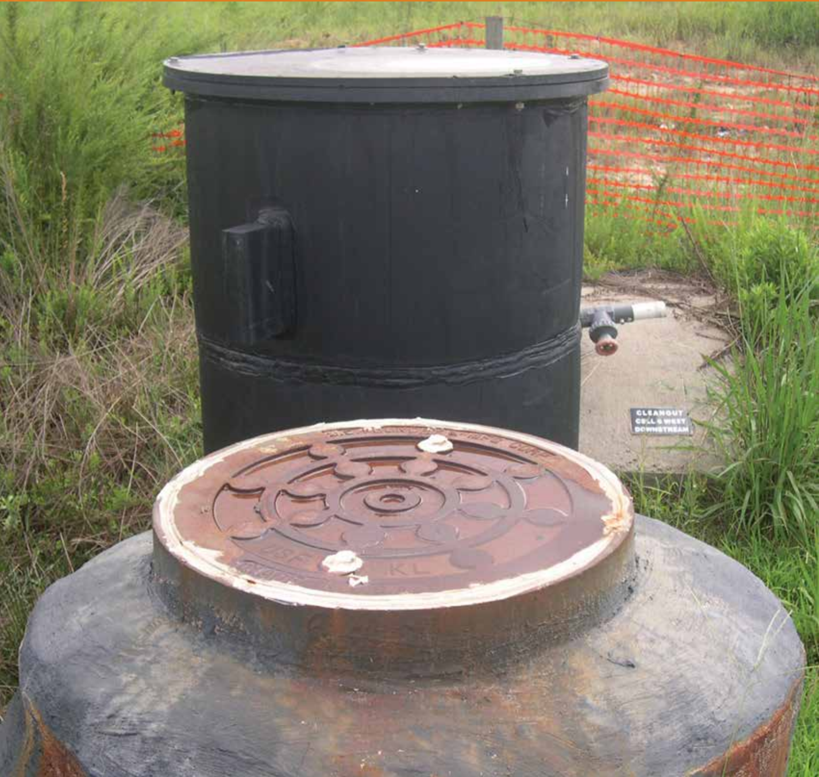
A leachate cleanout manhole at the Ann Street Landfill in Cumberland County, North Carolina. Regular maintenance of the leachate system is important for the success of a landfill gas project.
