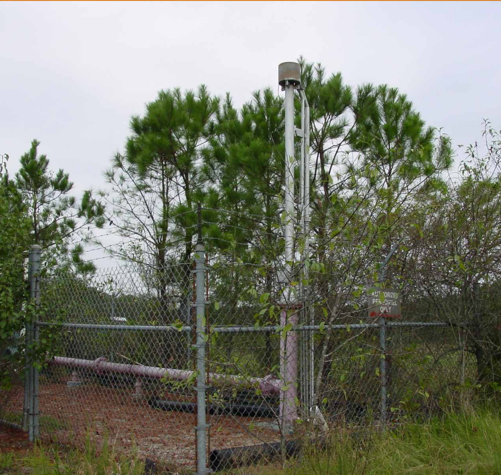
A landfill gas flaring system.
