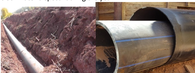
Laying of the sewer collector, dragging the pipeline DN1200 into the case under the road
