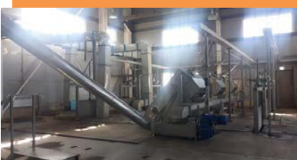
Sludge mechanical treatment equipment, installed in the bar screen building of biological treatment plants in Volzhsky
