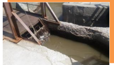
Emergency condition of sewage primary treatment facilities at the first stage of sewage treatment plants in Volzhsky before reconstruction
