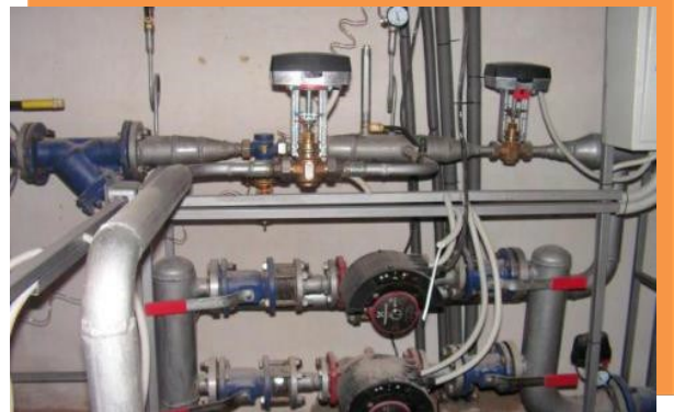
DHP equipment, installed in apartment building in Bratsk
