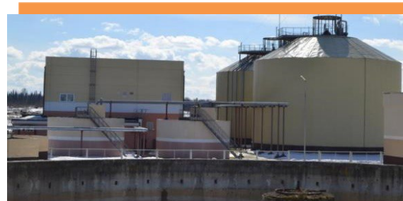
Methane-tanks (tanks for obtaining methane from a sludge) at the sewage treatment plants in Ivanovo
