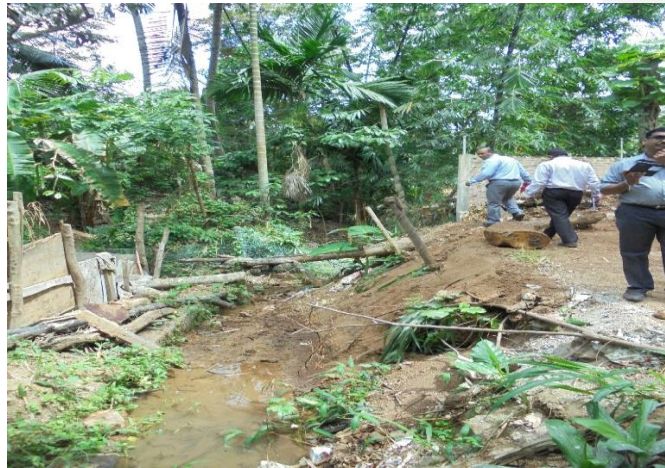
Heelpan-Kandura Stream with unprotected Banks in Residential Areas
