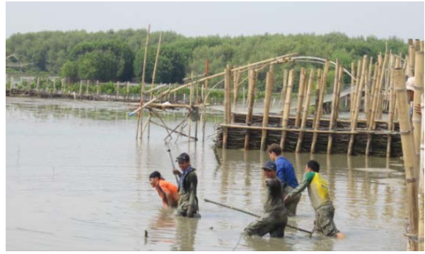
"Learning by Doing" – The community is trained to construct the permeable dams. (Source: Wetlands International)
