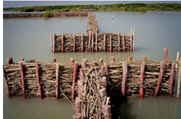
Permeable dams (Source: Wetlands International)
