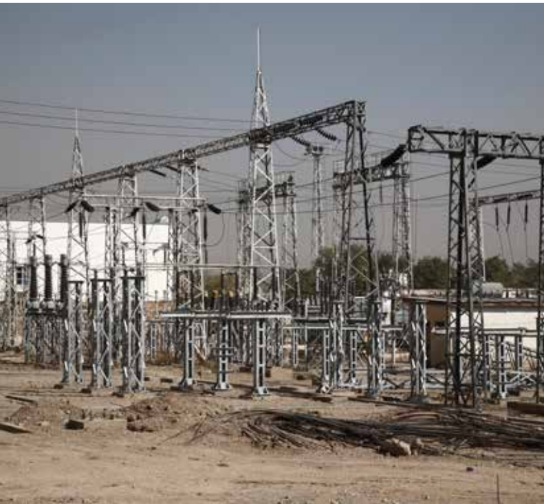
The North West Substation in Kabul. Photo: © Sofie Tesson / Taimani Films / World Bank
